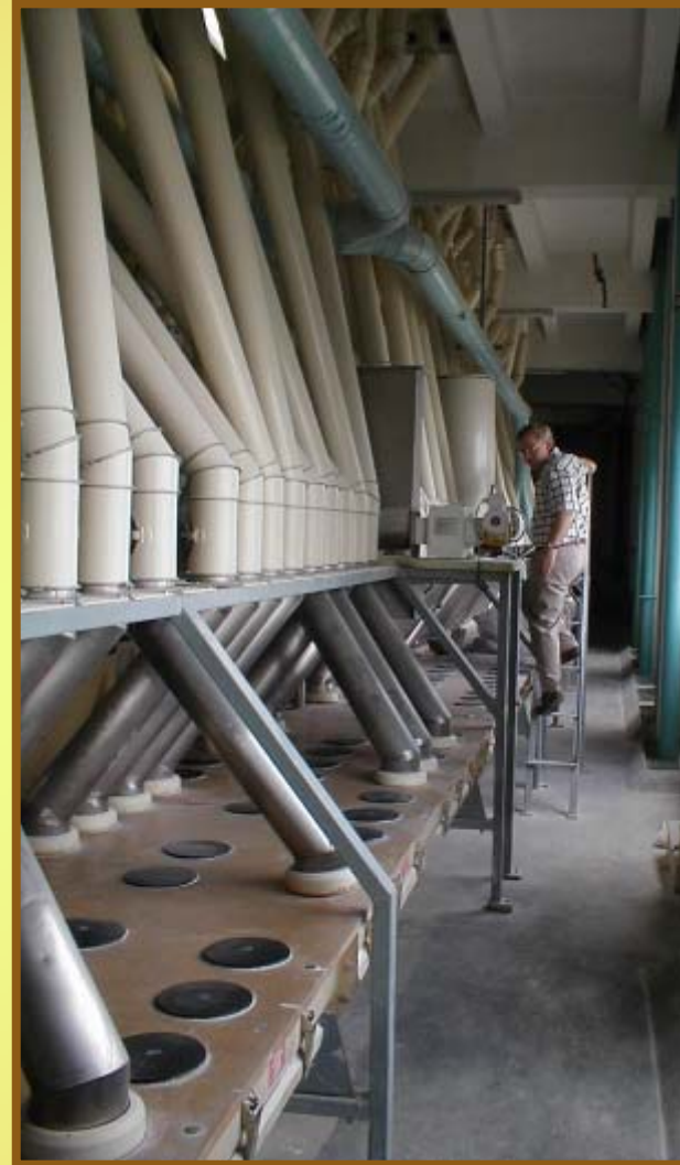
Flour collection conveyors for three different lines of flour. 面粉收集输送机用于三条不同的面粉线
