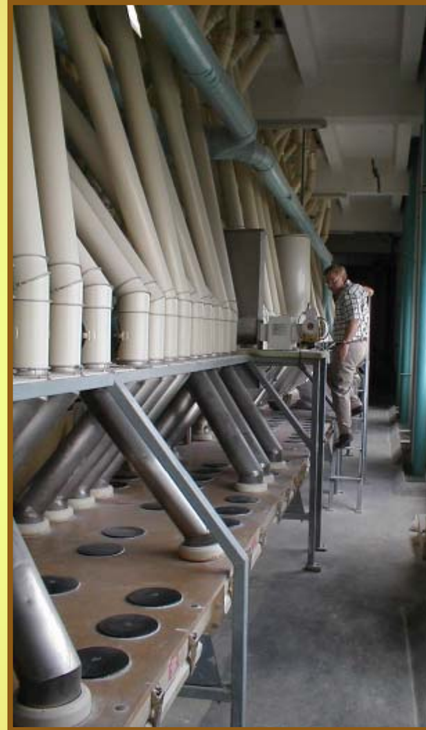
Flour collection conveyors for three different lines of flour. 面粉收集输送机用于三条不同的面粉线
